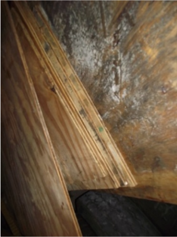
Plywood that does not conform to FBC 2007, no permanent hardware installed
