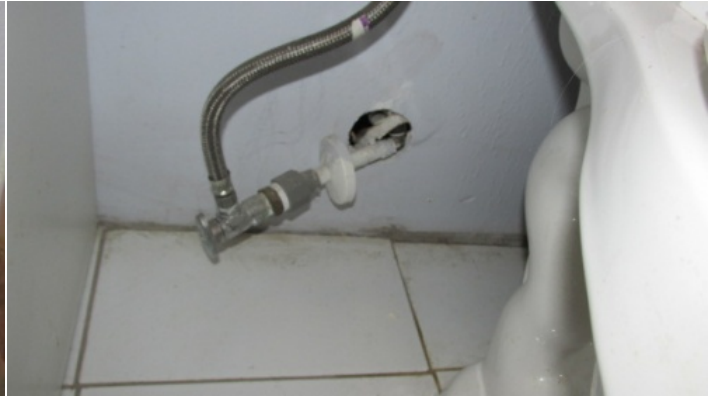
Toilet water shut off valve and flex metal water supply lines
