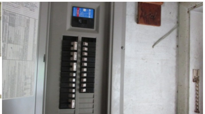
Circuit breakers - panel wiring looked good
