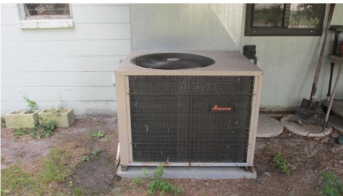
Heating & AC package unit
