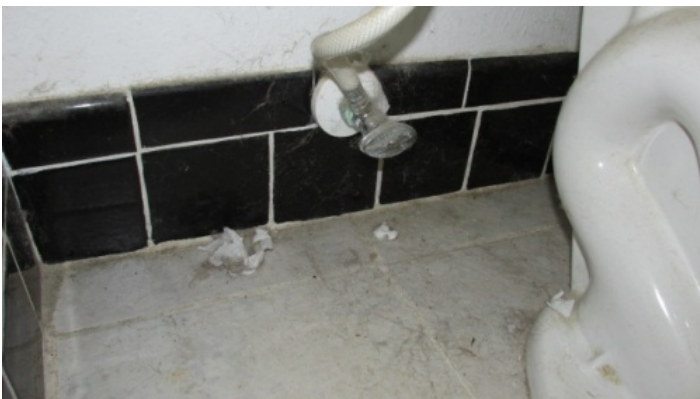
Toilet shut off valve
