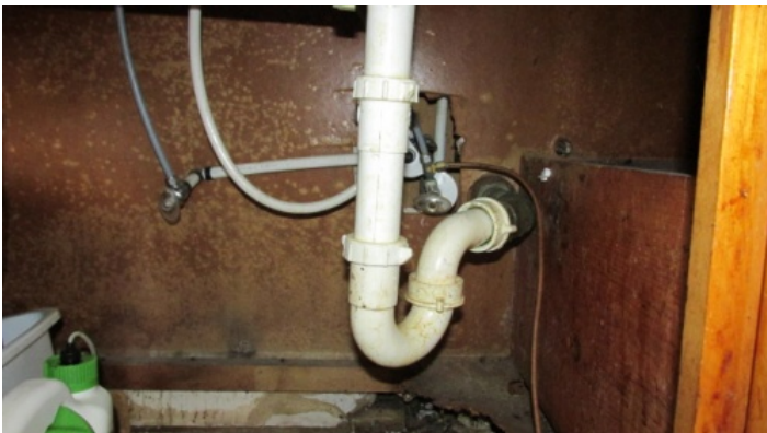
Kitchen Plumbing (under sink) - PEX water supply lines, PVC and galvanized drain
