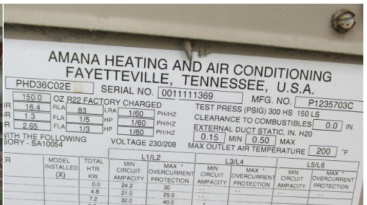
Heating & AC package unit label - mfg 2000
