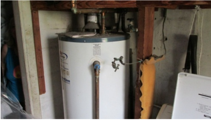
Gas water heater
