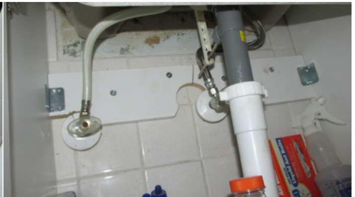
Bath Plumbing (under sink)
