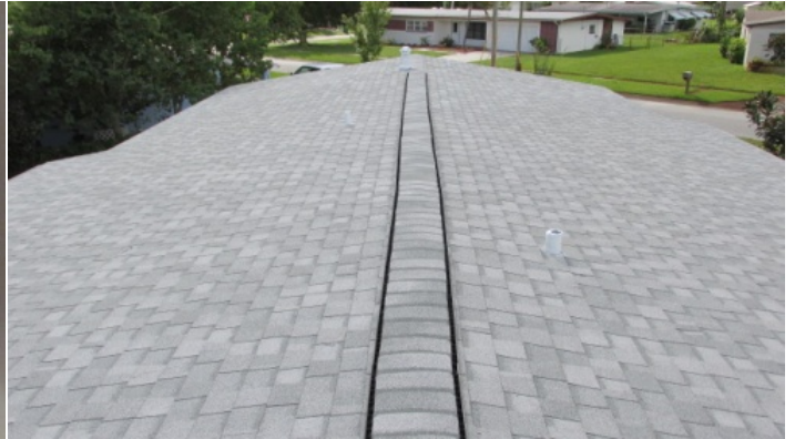
Roof ridge vent
